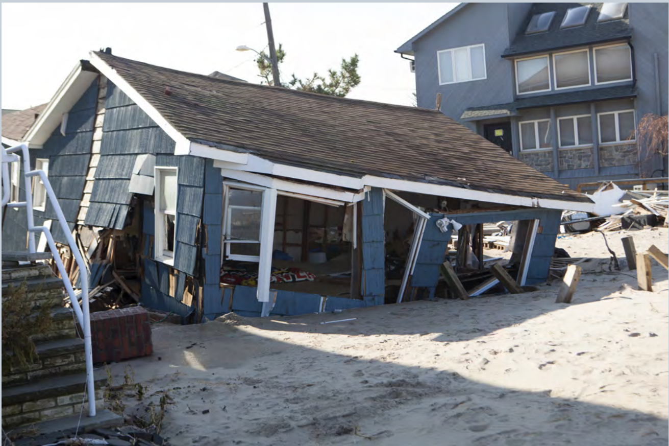
Destroyed homes during Hurricane Sandy in the flooded neighborhood at Breezy Point in Far Rockaway area of NYC, Nov 2012 (©AdobeStock)
